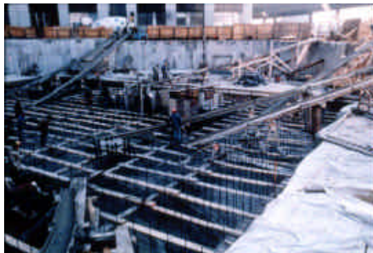
Fig. 9 - Placement of self-compacting concrete only chutes for the slab through foundation of the Trump Tower – New York (1978).
