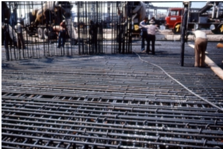
Fig. 6 - Congestion of reinforcement of a slab foundation where concrete (in the background) is placed without vibration [8].
