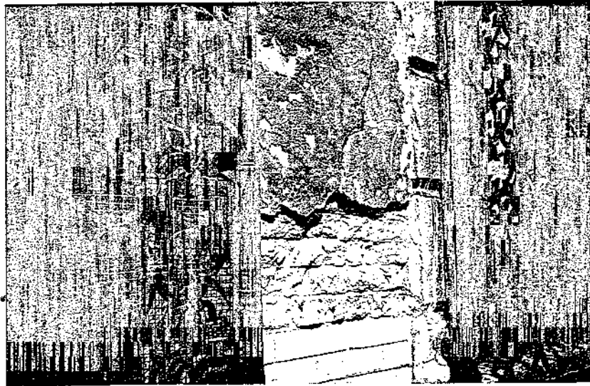
Fig. 11 Rendering mortar deteriorated due to the formation of ettringite. The mortar swells and falls out; however, residual rendering mortar is still coherent.
