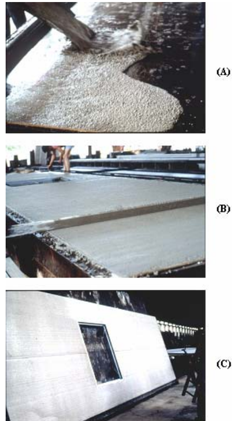
Figure 10. Precast lightweight concrete: casting of SCC (A); Screeding without vibration (B); demolding of the hardened lightweight panel (C).
